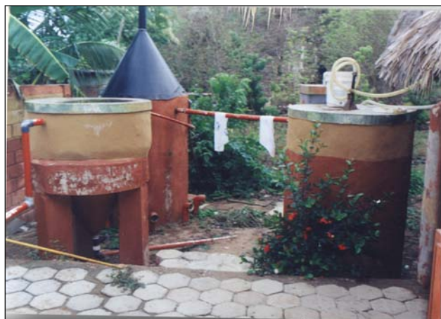
This biological treatment system in the organic cosmetic factory turns sewage into clean water without use of chemicals.
